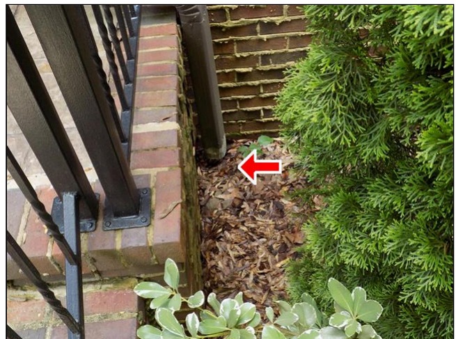
1.5 Item 9 poor drainage
