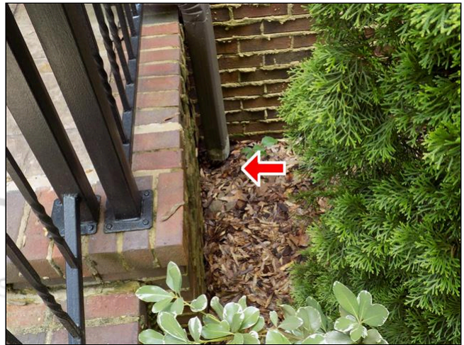
1.5 Item 9 poor drainage
